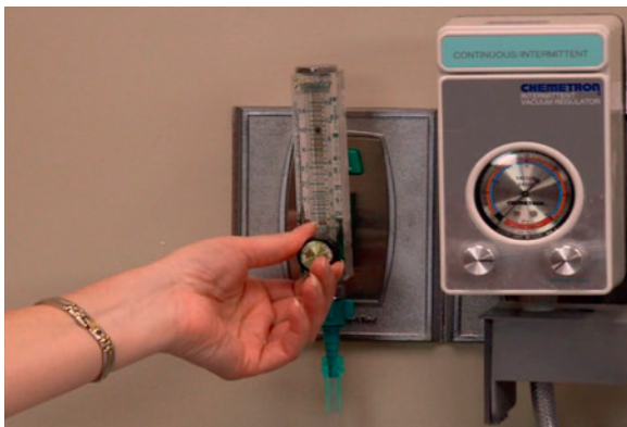
Fig. 50.2 Nurse adjusts flowmeter setting.
